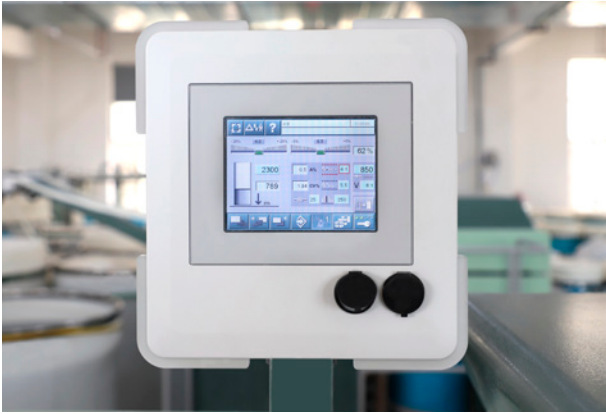
The RSB-D 50 is running at 850 m/min with recycled material at Wenzhou Luteng.
