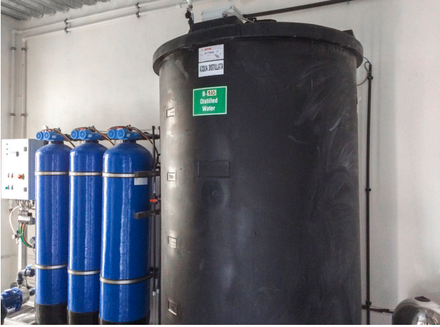
In Uzbekistan, the new wastewater treatment plant guarantees water reclamation of 90 to 95%.
